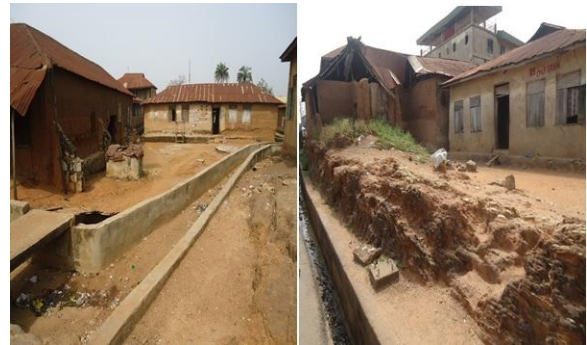
Figure 1: Deteriorated houses within the study area
